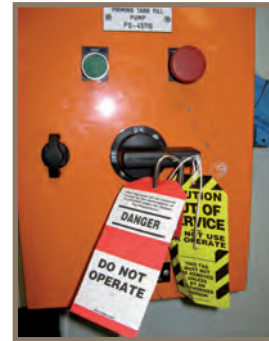
Tagged and locked switch
