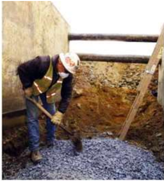
Pits, trenches gullies.
